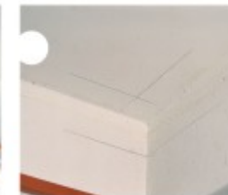
2. Marked on the wall and ceiling using the cornice to prepare for corner joints.
