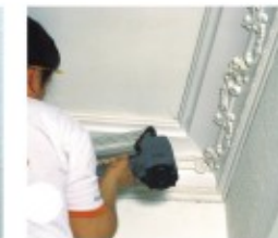
7. Fasten the cornice with the snail gun or steel snail, and fill the snail holes with plaster.
