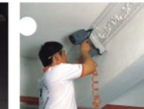
5. Using Pressure gun for snailing, if the wall is too strong use the steel snail.
